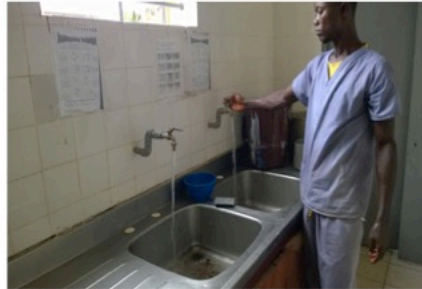
Taps with running water in the operating theatre
